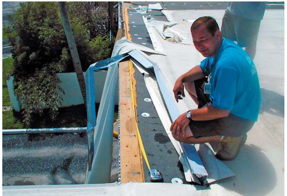
Charlotte County South Annex: Enhanced attachment of nailers and metal work would have likely allowed this roof to fare much better. Photo courtesy of RICOWI
